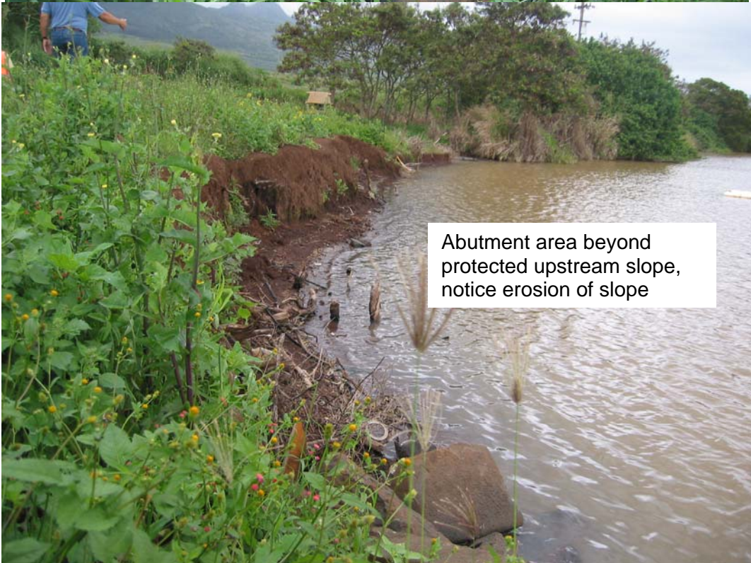
Downstream slope, only protected in the outlet works area, otherwise only heavily vegetated
